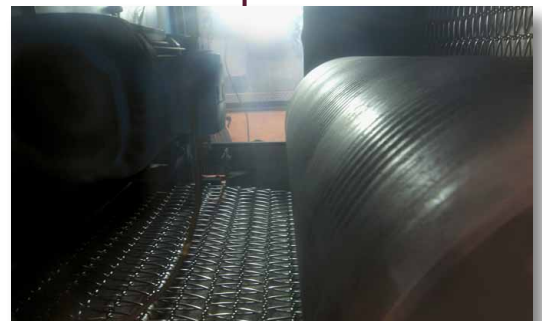
A look at the belt deflection facility
